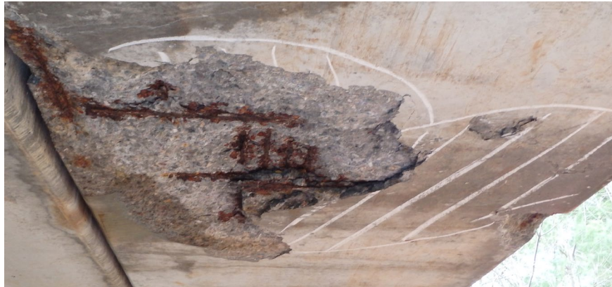
Figure 7.2.10-1: Example of Spalls and Delamination
